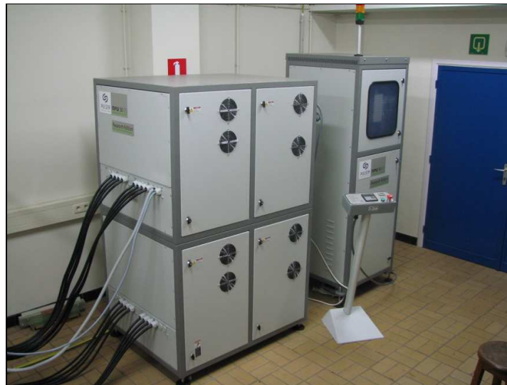
Figure 17 : Magnetic pulse equipment at BWI [9]
